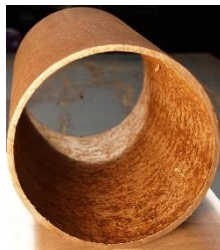
Figure 7. Corrosion of pipes due to the action of oxygen
