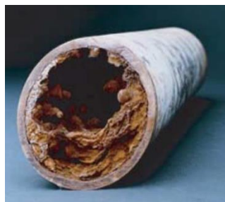
Figure 12. Microbiological induced corrosion
