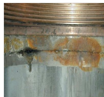
Figure 11 Corrosion damage caused by corrosion in gaps
