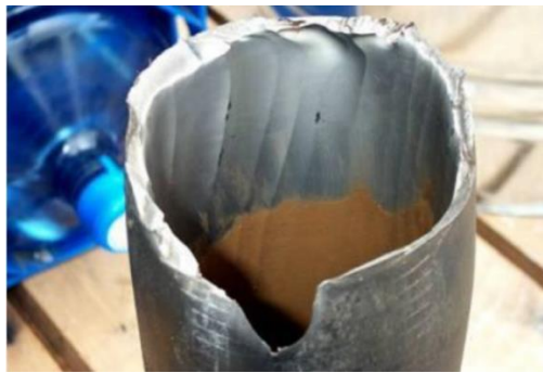
Figure 13. Fracture of pipes due to stress corrosion
