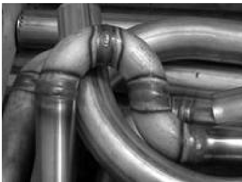
Figure 1. Heat tint in welded joints of a stainless steel.
