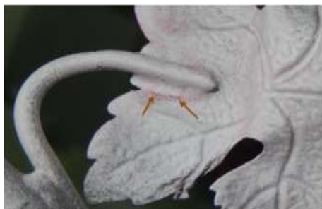
Figure 5. Enlarged view of discovered crack ( \approx 6\text{mm} in length) at leaf
