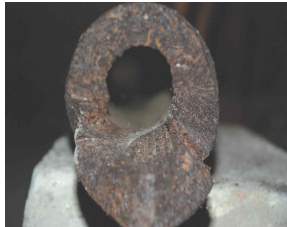
Figure 4. Photo of section in which there was a fracture of pipe.
